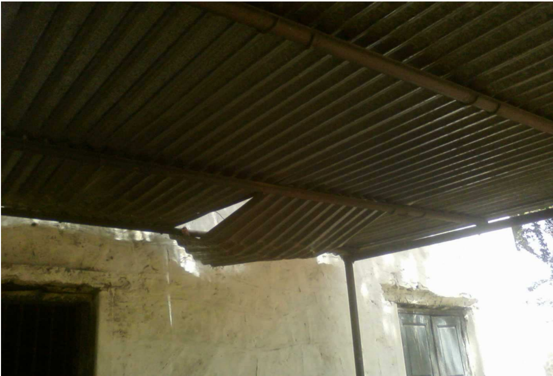
Pancha Primary School-damaged shed
