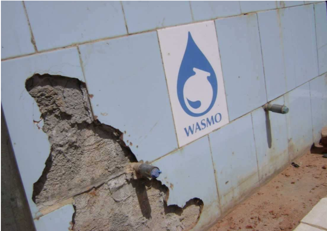
Captain Kalyan Singhji Primary School-Drinking Water Facility in damaged condition
