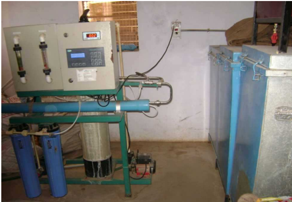
Lakhani Upper Primary School -R.O.Plant for Water Purification
